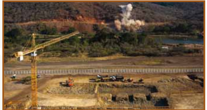
6 th Place / Photographer: DDP Photography ORO Projects: Lower Thukela Bulk Water Supply Scheme
