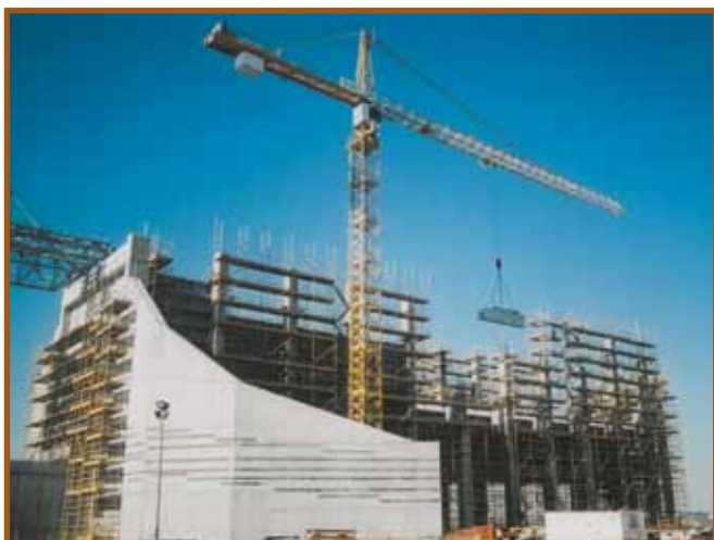
1 st Place / Photographer: J Jung Murray & Roberts: Material Handling System – Impumelelo Contract
